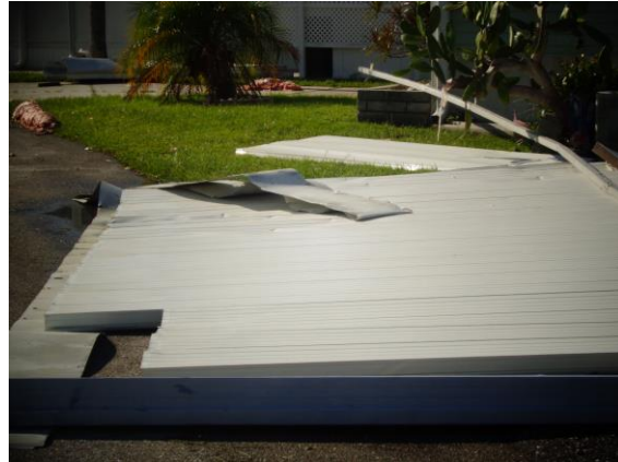
112 The roof over in the road
